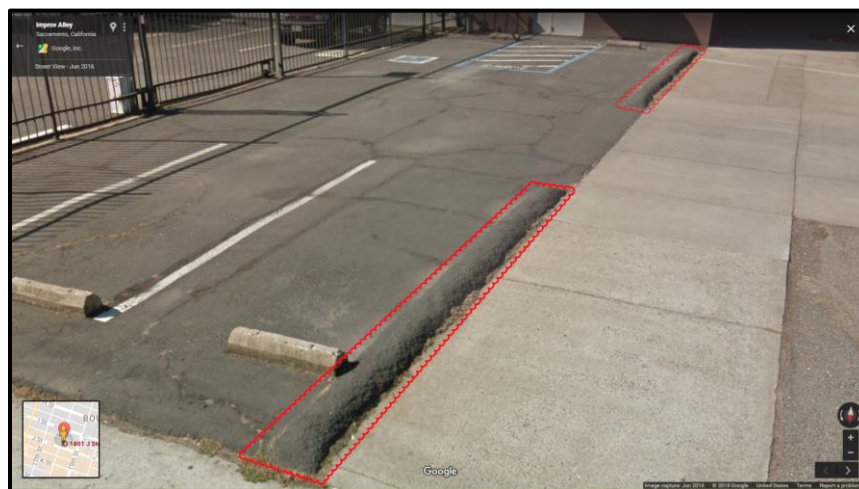
Figure 1 Asphalt berms next to the sidewalk
