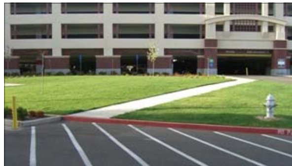
Walkway lacks curb cut
